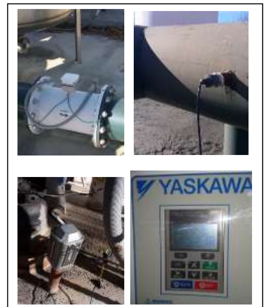
Figure 3. Magnetic flow meter (upper left), pressure transducer (upper right), acoustic groundwater level sensor (lower left), and VFD digital control panel (lower right).
