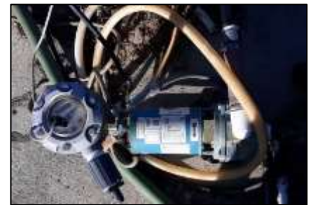
Figure 5. Pressure transducer on irrigation line (top) and flow meter on injection pump (bottom).
