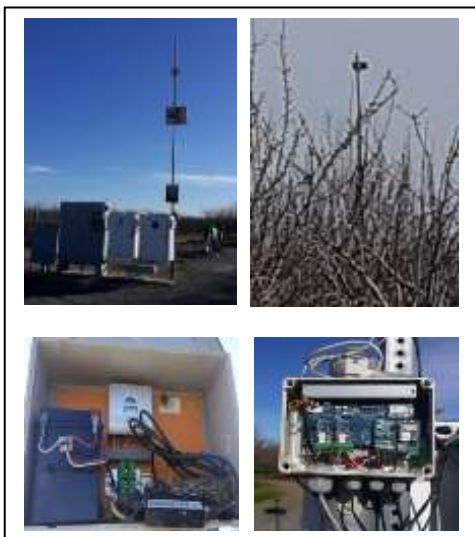
Figure 7. Parts of a telemetry system. Cell tower and gateway next to pump controls (top left), gateway connection to internet (bottom left), orchard cell tower connected to sensors in the field (top right); and node connection to field sensors (bottom right).
